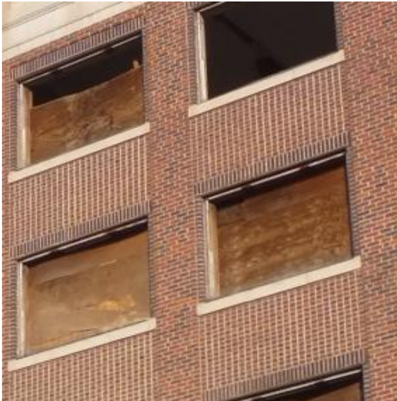
Photograph showing the stacked header bond below the windows and the pilasters.
